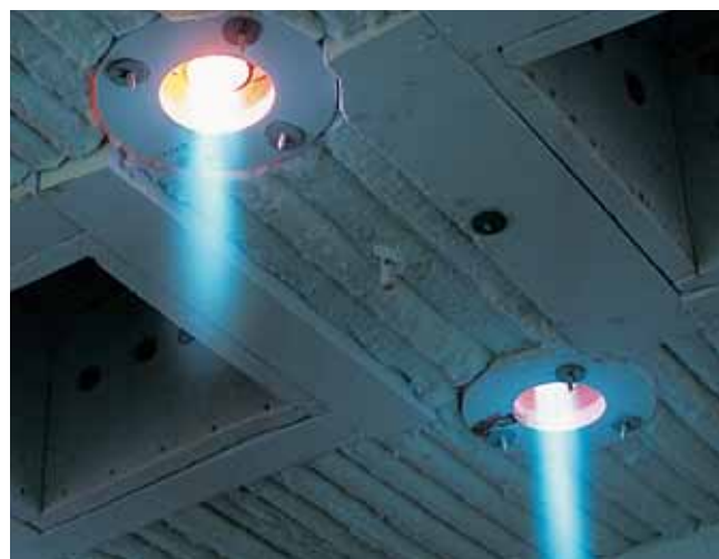
Roof-firing with BIC burners (Kromschroder)
